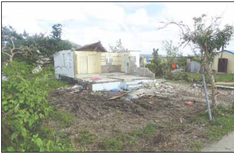
Category red: demolish and build new. Around 60% of buildings are with major structural damage.
